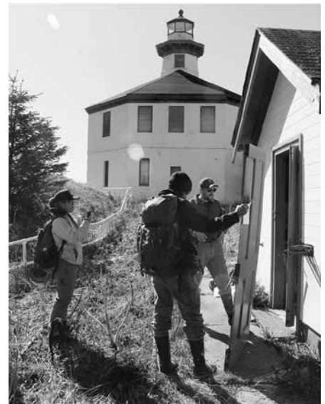
Sue York, Eldred Rock Lighthouse Preservation Association executive director, and board members Justin Fantasia and Jonathan Wood examine a broken door at the lighthouse in April 2019. Photo by Alex McCarthy, Juneau Empire.
