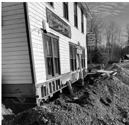
New owners had started repairing the historic Fairview Inn prior to the earthquake this fall.
