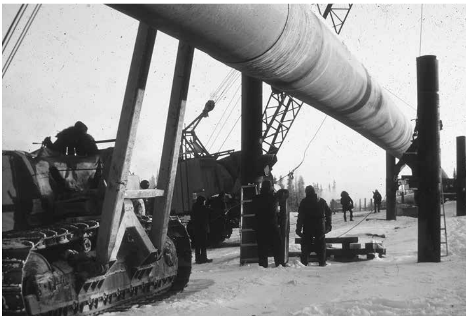
Trans-Alaska Pipeline workers place pipe on vertical support modules. The balance between resource development and conversation has long dominated Alaska public policy. UAF-1990-129-65, Mumby Trans-Alaska Pipeline Slides. APRCA, University of Alaska Fairbanks.
